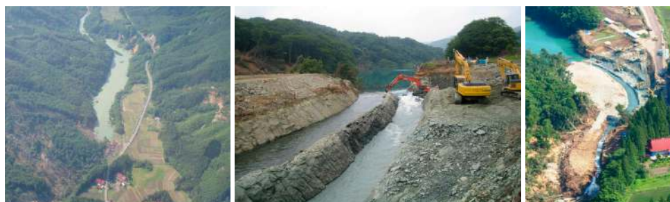
The Iwate-Miyagi Inland Earthquake; 2008, Iwate and Miyagi Pref., Japan (Construction of an emergent drainage channel to lower water level; Just after earthquake; Countermeasures completed)
