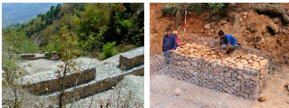
Series of Gabion sabo dams; Dahachowk, Nepal
